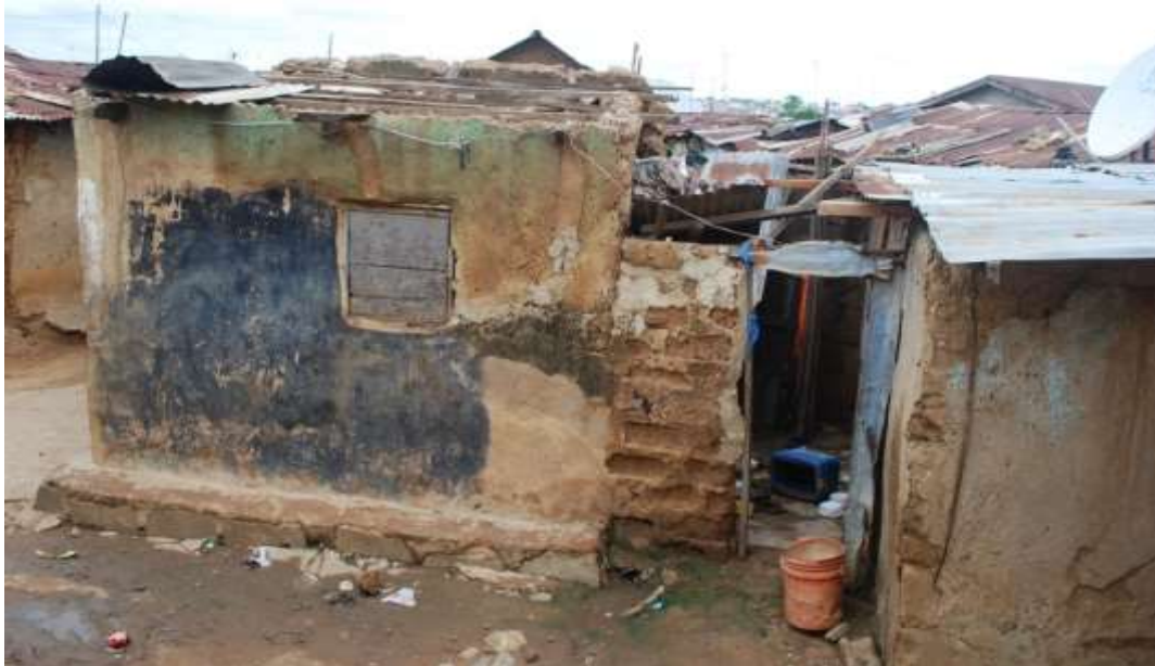
Plate 2: Poor Roofing Condition in Down Quarter
